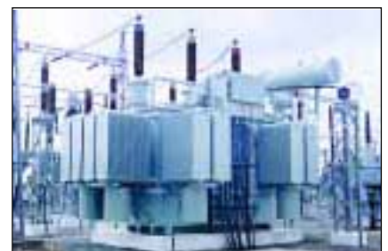
30 MVA, 110/33 kV Transformer with Ashburton, New Zealand
