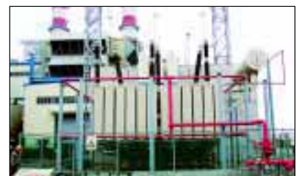
320 MVA, 16/230 kV GSU Transformer with AES Haripur 450 MW Power Plant, Bangladesh
