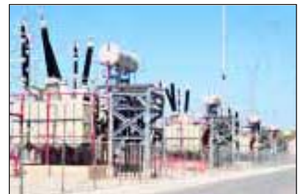
120 MVA, 13.8-13.8/345 kV Generator Transformers with 900 MW Macaè Merchant Power Plant, Brazil
