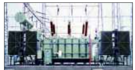
315 MVA, 400/220 kV Auto Transformer with NTPC, India
