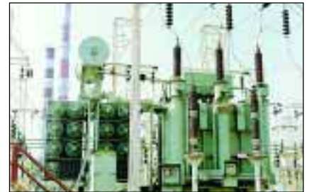
90 MVA, 11/132 kV GSU Transformer at TATA Power in India.
