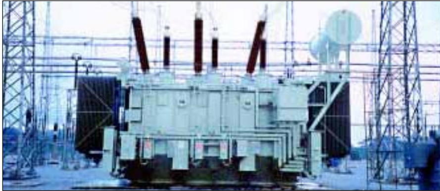
240 MVA, 275/132 kV Auto Transformer with TNB, Malaysia
