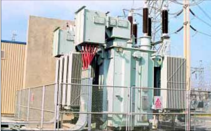
77/96/110 MVA, 11.5/115 kV, GSU Transformer at Rojana & Saha Co-Gen, Thailand
