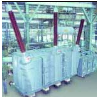
315 MVA, 420/220 kV Auto Transformer in 1984
